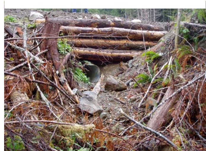
Logs do not fully retain road fill above a small stream.
