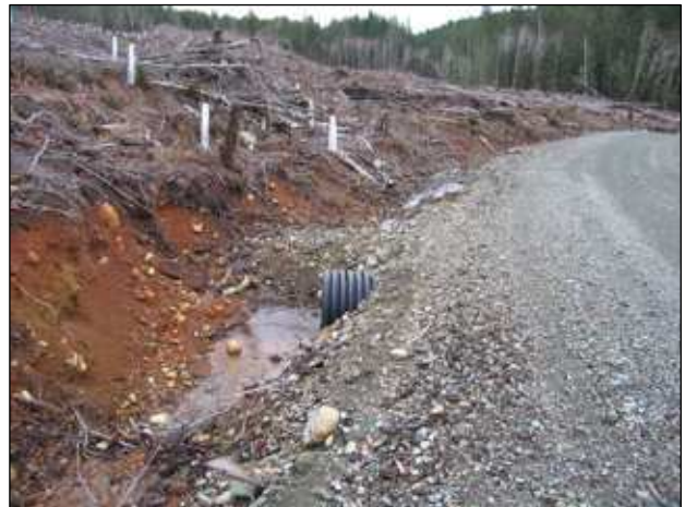
10. Culvert ditch block, and ditch cleared after harvest to prevent road fill encroaching.
