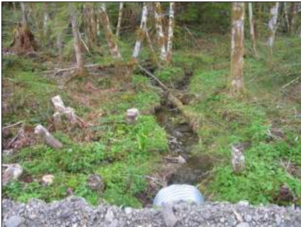
3. Natural drainage pattern maintained.
