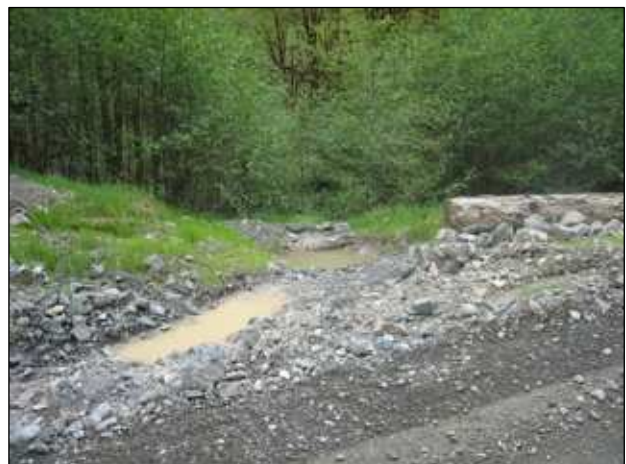
6. Settling basins in ditchline can be cleaned out periodically to help to reduce risk of sediment delivery.
