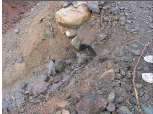
2. Culvert too short and outlet partially plugged.
