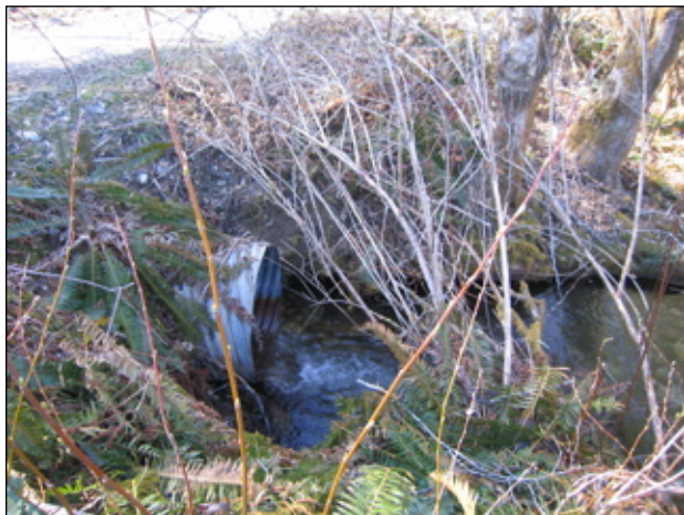
16. Legacy road issue – perched culvert outlet on fish stream.
