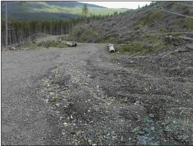
7. Looking down-grade. Note rill erosion caused by ditch water discharging onto running surface of road.
