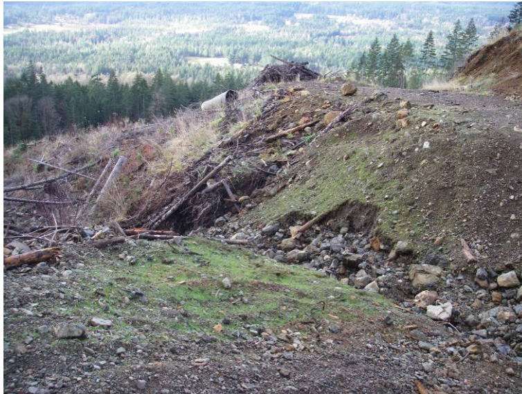
FIGURE 4. C23. NOTE SLUMPING ALONG THE BANKS OF THE CROSS-DITCH. THIS DITCH SHOULD HAVE HAD A STEEPER GRADIENT, BUT IT SHOULD NOT PRODUCE SUBSTANTIALLY MORE SEDIMENT. NOTE THE SEEDING ON THE OUTSIDE OF THE ROAD. COVER WILL LIKELY INCREASE NEXT YEAR.
