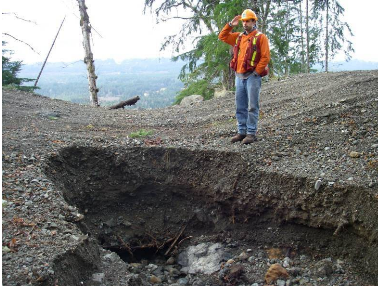
FIGURE 6. EROSION AROUND PIPE INTAKE (THE INTAKE IS AT THE BOTTOM OF THE HOLE) AT CROSSING C18. THE PIPE SHOULD HAVE BEEN REMOVED IN DEACTIVATION AND THE ORIGINAL CHANNEL GRADIENT RESTORED, BUT THIS HAS SINCE BEEN DULY COMPLETED (D. IANNIDINARDO, PERS.COMM).
