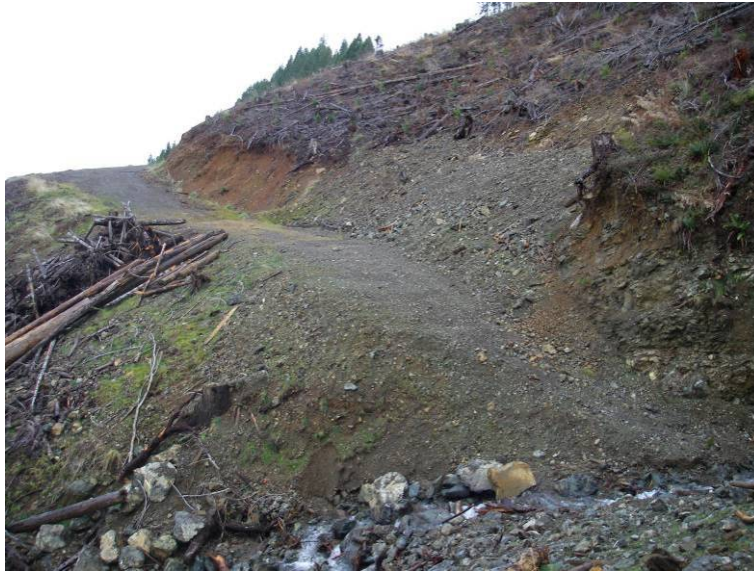
FIGURE 3. C27 CROSSING LOOKING TOWARDS THE NORTHWEST. THE CROSSING HAS BEEN RESTORED TO NATURAL CONFIGURATION AND SPOIL WAS PULLED AND PLACED AGAINST THE CUT. THE CROSSING HAS BEEN ERODED BUT IS NOW PROPERLY GRADED AND SHOULD NOT PRODUCE SUBSTANTIALLY MORE SEDIMENT.
