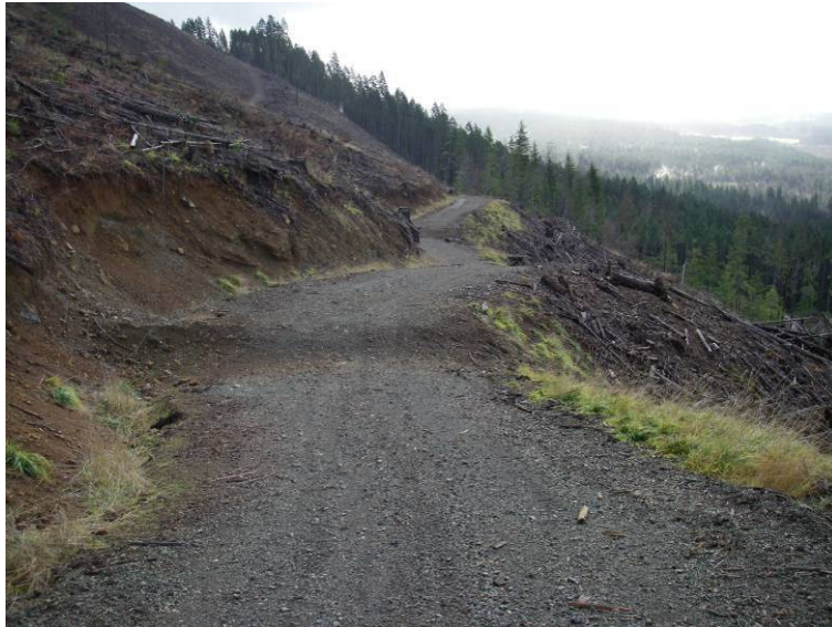
FIGURE 2. ROAD BETWEEN C1 AND C27. DEACTIVATION IS APPROPRIATE AND HAS SUCCESSFULLY WEATHERED ITS FIRST YEAR. SEEDING IS ADEQUATE.
