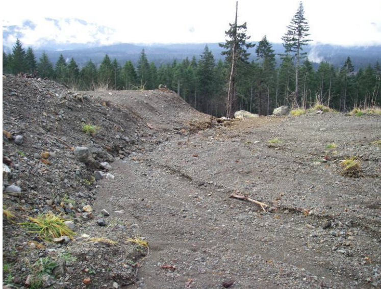
FIGURE 7. LOOKING DOWNSTREAM AT C11. TIMBERWEST HAS EXCAVATED A CROSS-DITCH AND INSTALLED A BERM ON THE DOWN-GRADE (LEFT) SIDE. SOME EROSION IN THE FORM OF RILLING HAS OCCURRED ON BASE OF THE DITCH; THIS IS A RELATIVELY MINOR SOURCE OF SEDIMENT. THE CULVERT REMAINS IN PLACE, SO IT SHOULD BE MONITORED FROM TIME TO TIME.
