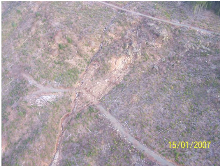
FIGURE 1. CULVERT ON SPUR 200 AT STREAM 7. IN THIS PICTURE IT IS FUNCTIONING ADEQUATELY.
